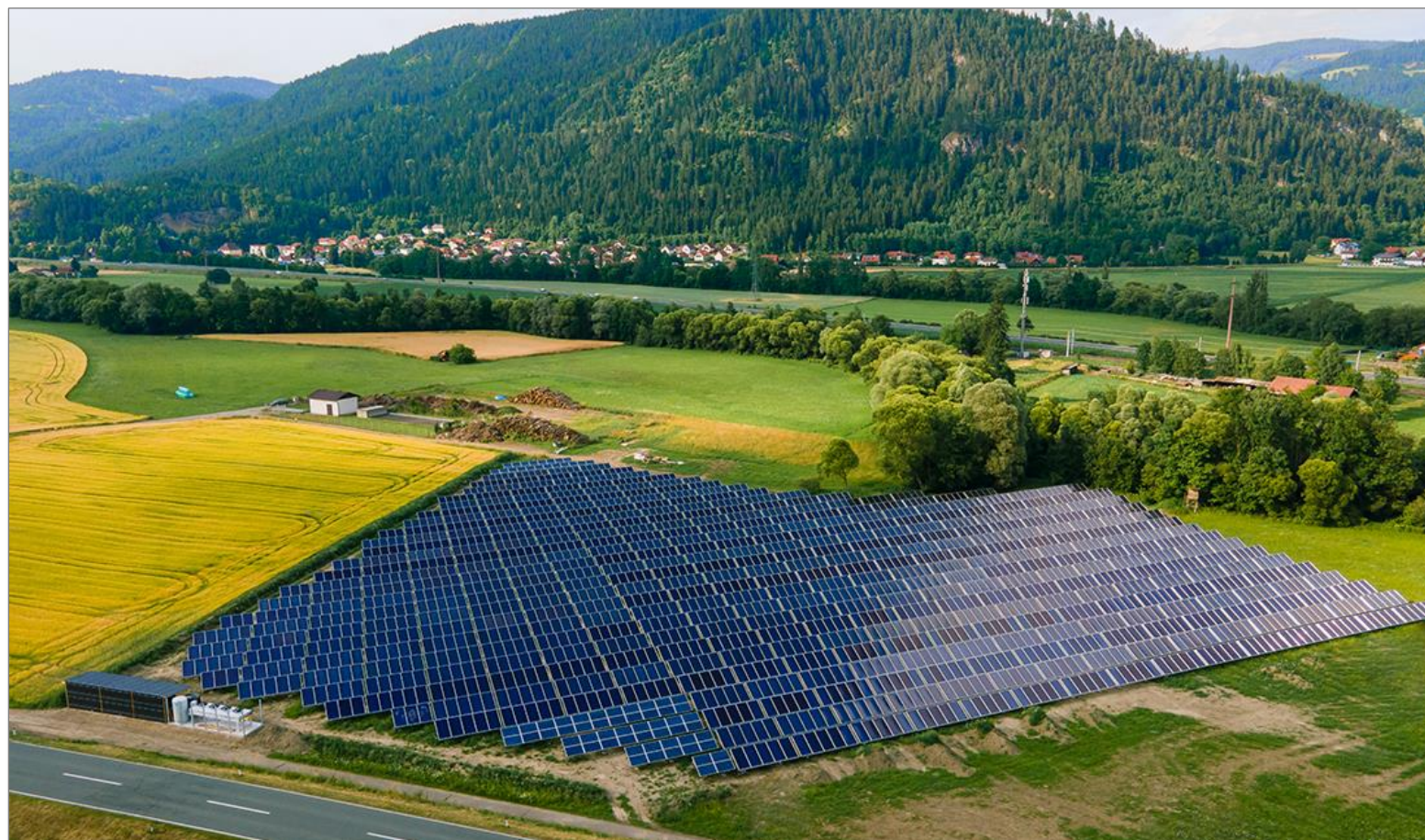
Friesach, Source: Solar Engineering Guggenberger
