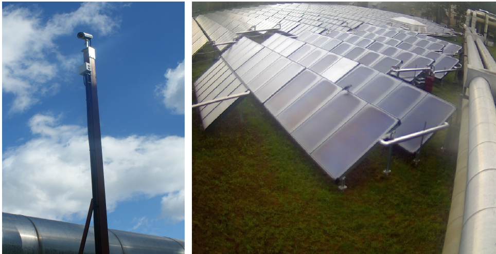
Figure 12: Mounting of webcam at FHW plant (left) and sample picture (right).
