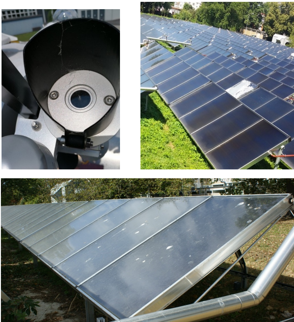
Figure 17: Soiling of pyrheliometer in winter (top left), broken glass of collector shortly after inauguration (top right), soiled collector (bottom).
