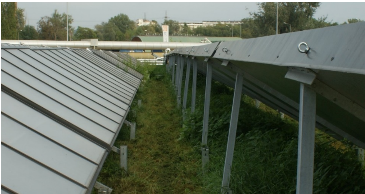
Figure 7: Collector mountings at the FHW plant.
