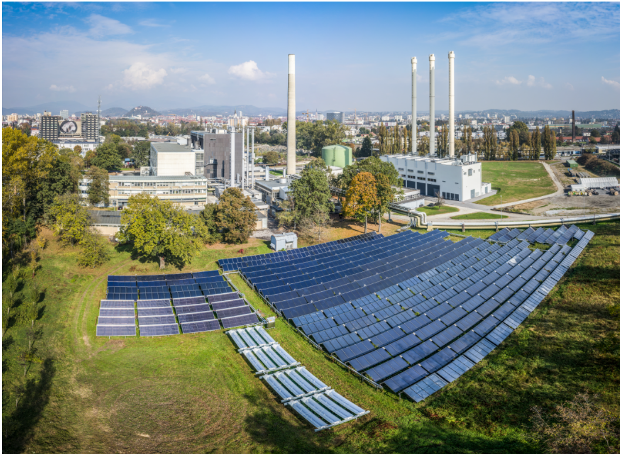
Figure 6: Collector array of FHW plant with ground-mounted collectors. Source: SOLID, Picfly.at Thomas Eberhard.
